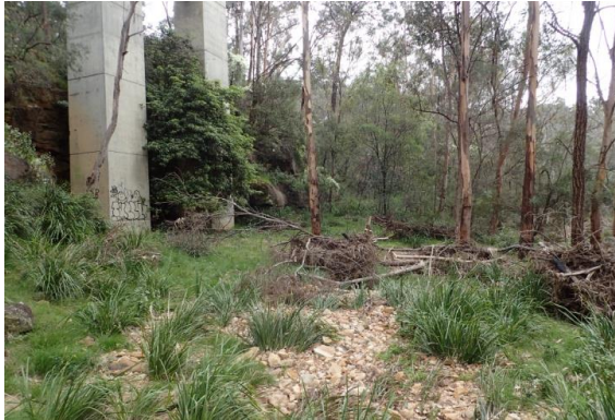
Plate 5. View to west, Moolgun Creek Bridge. This level area next to Allens Creek had been inundated from recent flooding. Pylons at left had been fitted into a cavity cut into sandstone bedrock.
