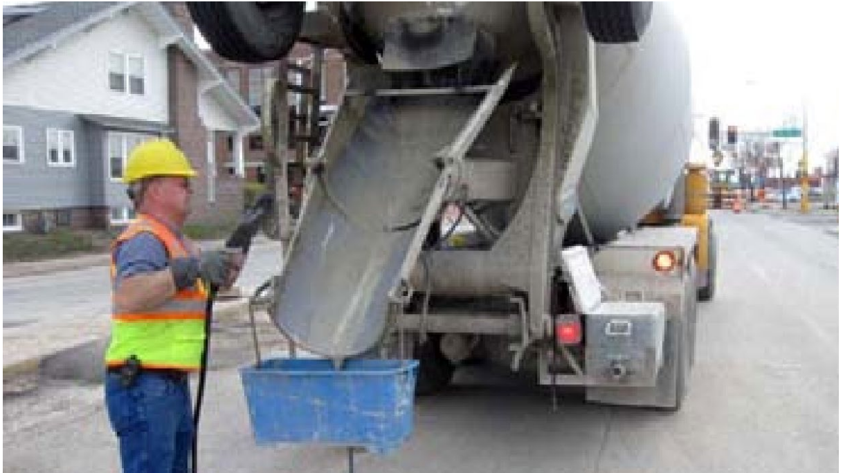
Photo: Minnesota Dept of Transportation, Best Management Practices for Concrete Washout , 2009, version 5
