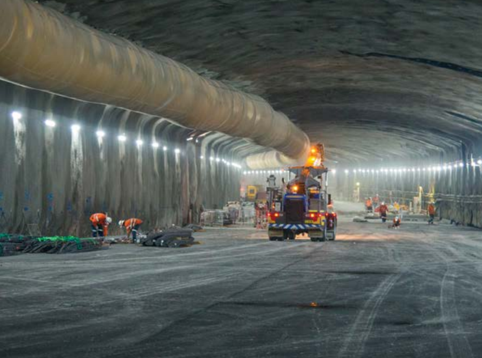
Work on the New M4 Tunnels ahead of their opening in mid-July 2019.
