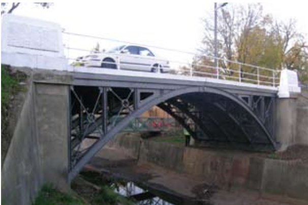
Recently repainted historic iron arch bridge over Bungambrawatha Creek (built in 1886) on Riverina Highway.
