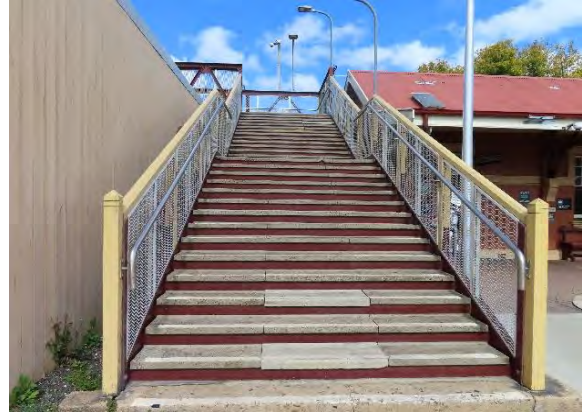
Figure 5.22 View of the stairway to the western side of the Argyle Street footbridge.
