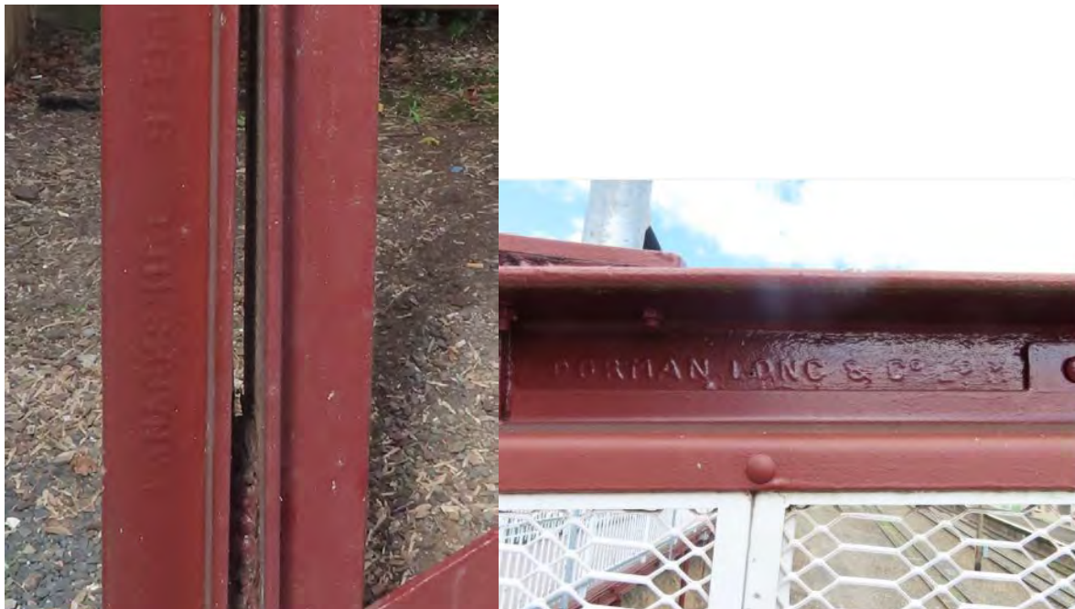
Figure 5.18 Foundry names of Lanarkshire Steel and Dorman Long embossed on steel trestle posts on the original components of the footbridge. (Source: GML 2023)
