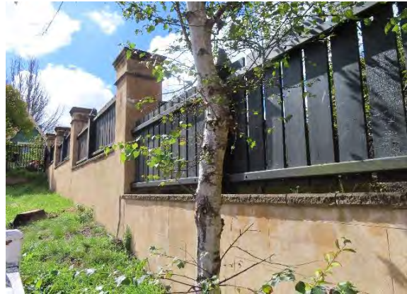
Figure 5.6 The sandstone wall along the western side of the former Post Office building, adjacent to the footbridge.
