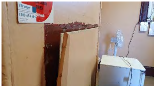
Figure 4-10: A4 SSER Room, Building A (AECOM, 2023)
