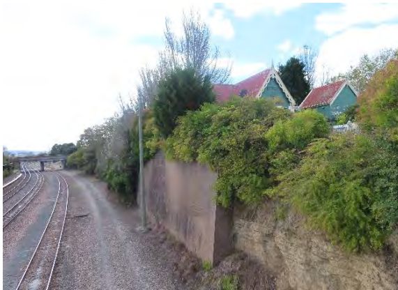
Figure 5.27 View of the Station Master's residence, the embankment and the brick retaining wall looking northeast from the footbridge.
