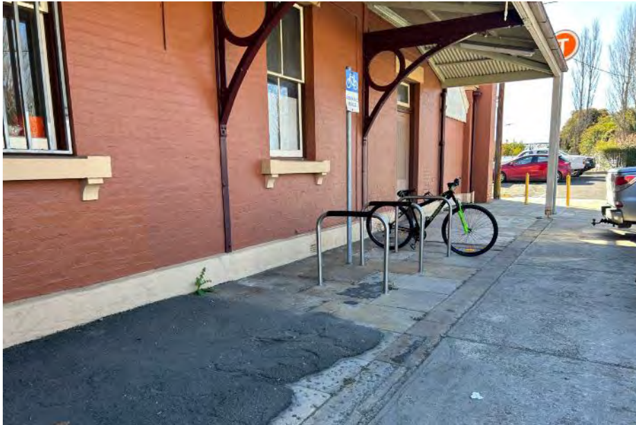
Figure 8-11: Sandstone flagging partially covered with bitumen beneath the eastern awning of Building A, facing the forecourt and car park (AECOM, 2023)
