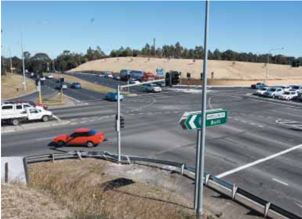
Pinch Point Program: Completion of intersection upgrade at Narellan Road, Blaxland Road and Gilchrist Drive at Campbelltown.
