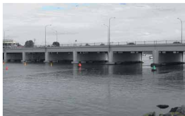
Endeavour Bridge after concrete repair work, cathodic protection of reinforcements and application of anti-carbonation coatings work.
