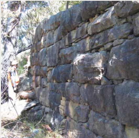
A remaining section of the heritage item retaining wall, built in the 1840s from formed sandstone, standing over 2.2m in height.
