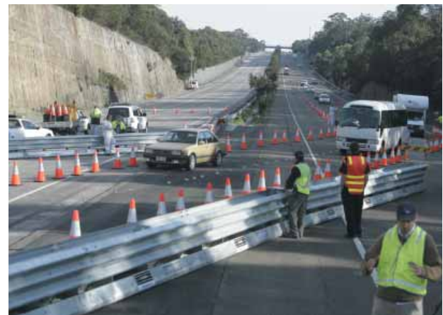
The RTA and NSW Police Force conducted a major training exercise on the F3, Sunday 26 October, under live traffic conditions to train for the implementation of a contra-flow on the F3 Freeway between Ku-ring-gai Chase Road and Pacific Highway Wahroonga.
