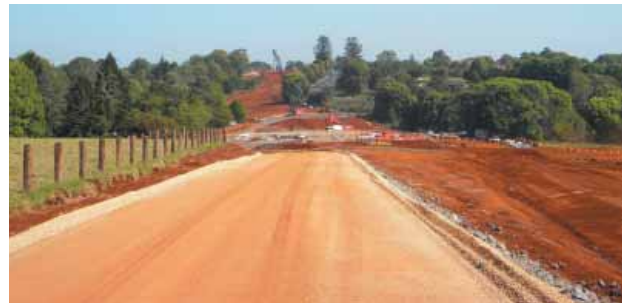
Construction works at the Alstonville Bypass, expected to be completed in late 2010.
