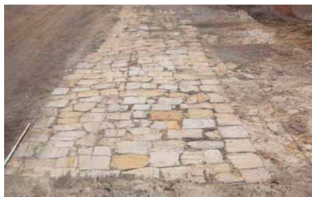
View of sandstone block road base c.1860 exposed and recorded at Leura during duplication works for the Great Western Highway in December 2008. Ref: Final Archaeological Report – Great Western Highway, Leura-Katoomba, Stages I, II and III. Archaeological Management and Consulting Group Pty Limited, March 2009.
