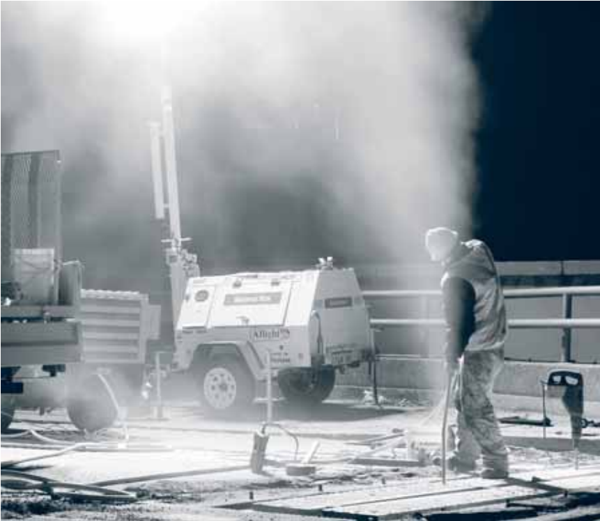
RTA Bridge Services – civil crew undertaking night works on the Cahill Expressway to replace expansion joints.
