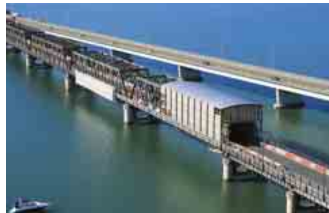
To help manage traffic issues, lead and asbestos contaminants and OHS risks, the team repainting Tom Ugly's Bridge devised an innovative containment structure to protect staff and contain contaminants.
