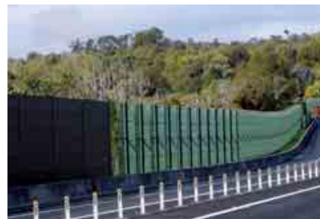
This noise wall along the Pacific Highway at Ewingsdale is just one of the measures the RTA uses to reduce highway noise.
