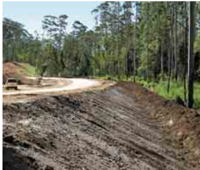
Mulch bank for sediment control along a road at Bonville on the North Coast of NSW.
