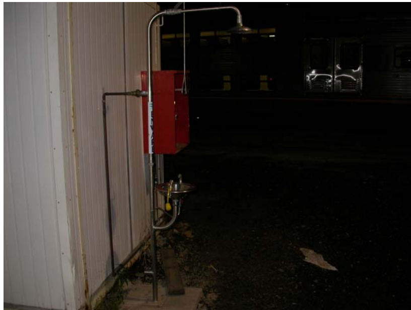
Typical Enware Emergency Shower and Eye Wash (Penrith yard)
