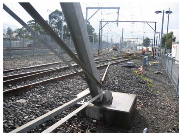
Catch point in an undesirable location
