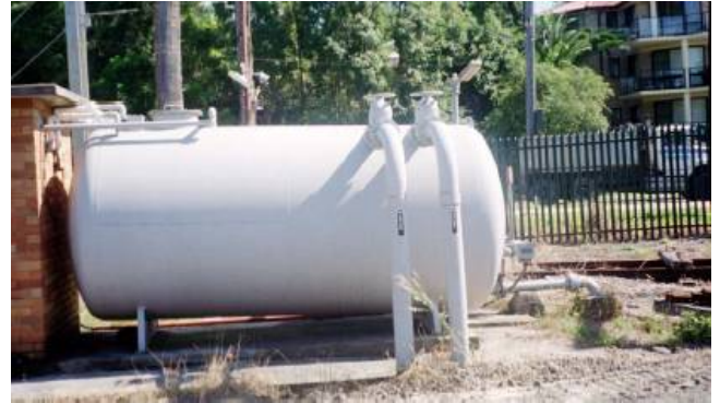
Gosford Decanting Facility
